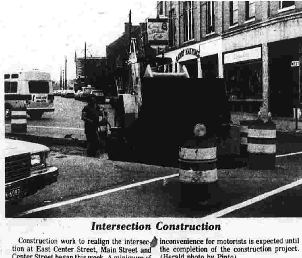
Construction work to realign the intersection at East Center Street, Main Street and Center Street began this week. A minimum of
